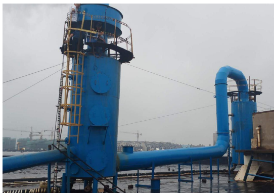
焙烧炉二级塔喷淋
